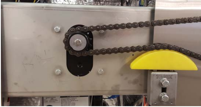
Obsolete Spring-Loaded Chain Tensioner
